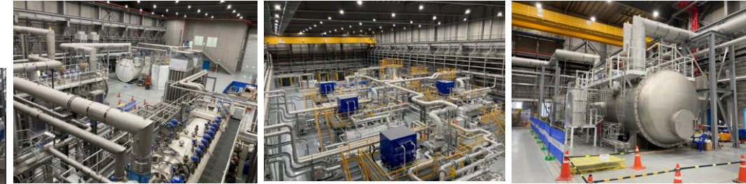
Cold box Warm compressors LHe Dist. box
